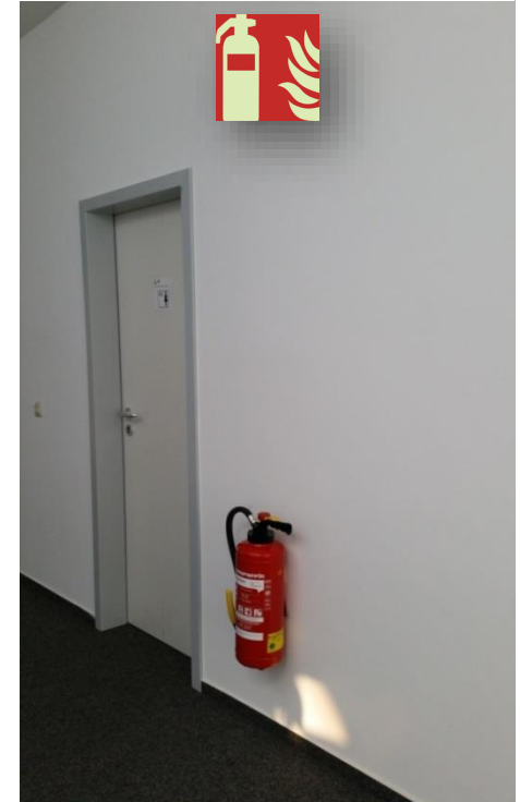
Fire extinguisher everywhere
